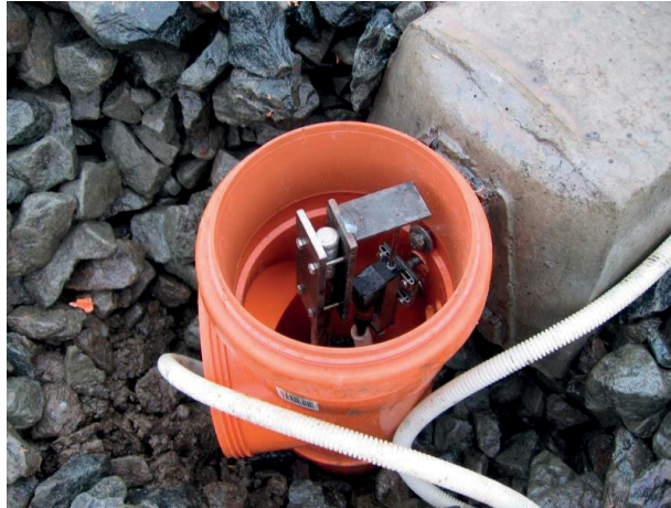
Figure 3.16. Measuring system built to measure frost heave in the structural layers of a track.
