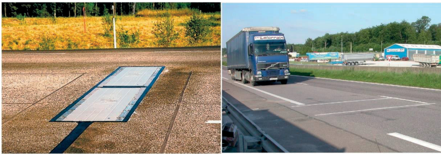
Figure 2.16. Two WIM stations: bending plates on the left and piezo-ceramic strip sensors on the right (Jacob & Feypell-de La Beaumelle 2010).
