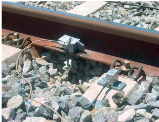
Figure 2.21. Accelerometer sensors installed on the foot of the rail and on the sleeper head in connection with the SUPERTRACK project (Supertrack 2005).
