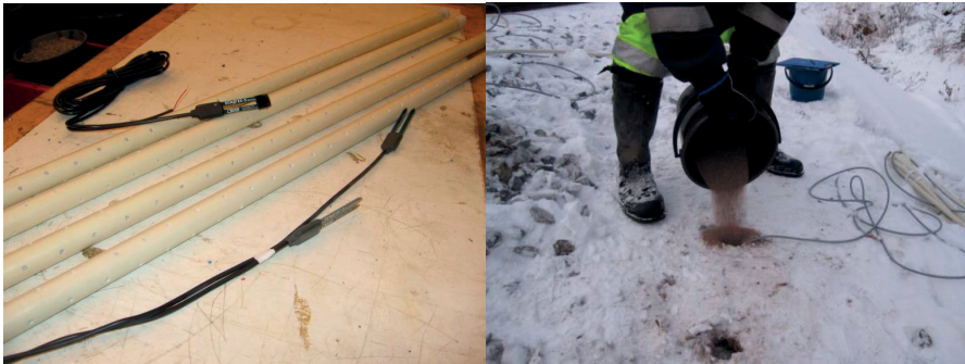
Figure 3.41. Water content sensors, ready-to-install sensor elements and the installation hole being filled with sand.
