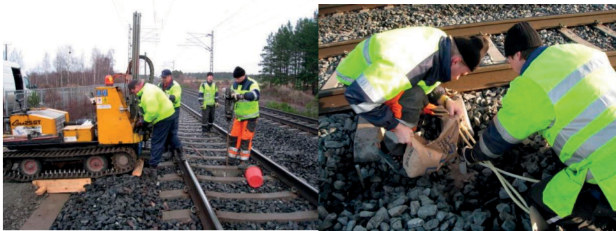
Figure 3.10. Installing MDD. The sensor element was installed in a 50-mm hole made with a drill rig (on the left) and fixed to its surroundings with installation sand (on the right).
