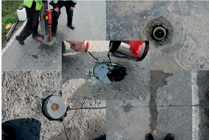
Figure 3.11. Some of the installation phases of a sensor measuring deflections in the pavement.
