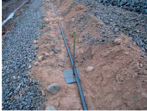
Figure 3.35. One of the embankment settlement's measuring points for levelling.
