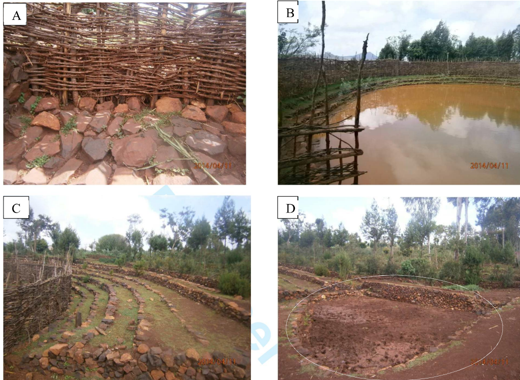
Figure 4. (A) Wooden mesh to filter debris coming to the pond, (B) Fenced pond, (C) Outside terracing to protect silt from the sides of the pond, and (D) Stilling basin that settles silt coming in with flood before entering the pond. (photo by Behailu April, 2014)
