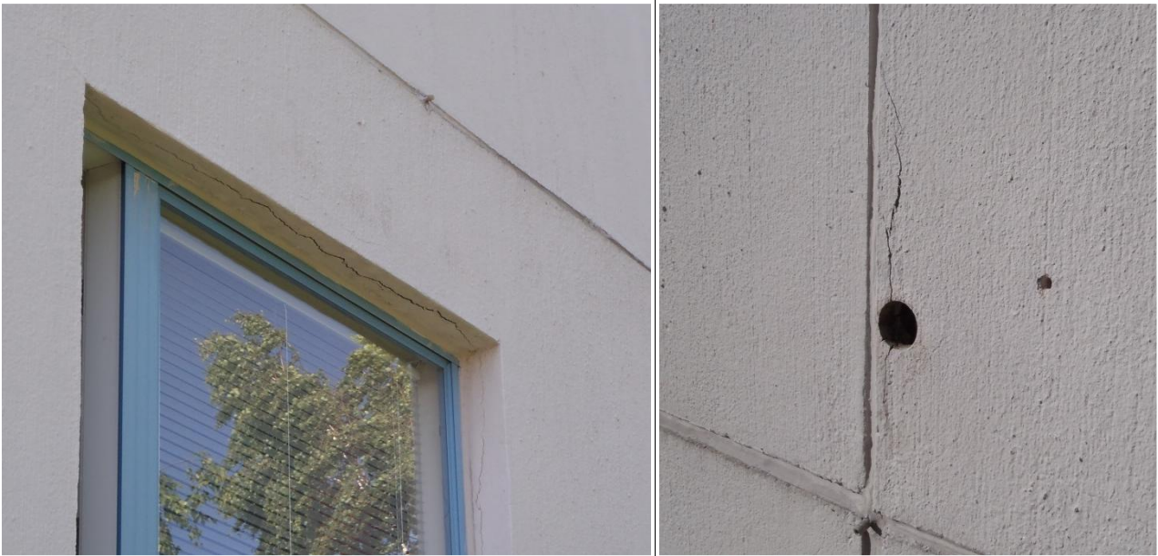
Figure 1.3 Typical corrosion damage on concrete facades
