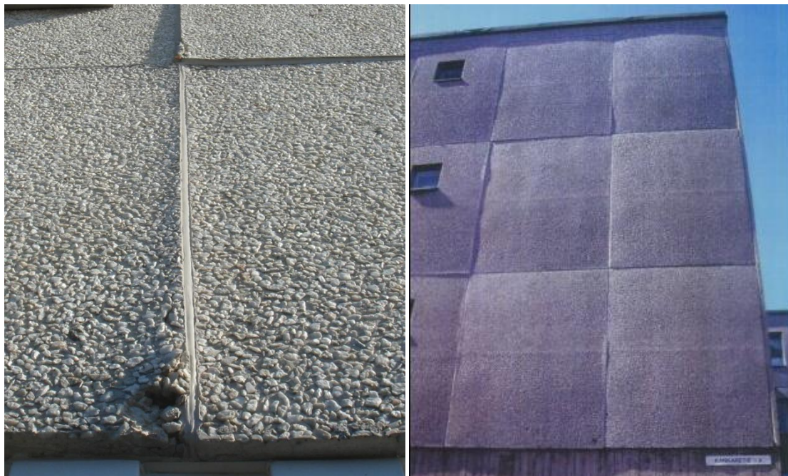
Fig. 5.24 On the left, local frost damage at the edge of an exposed aggregate concrete panel. On the right, far advanced and wide spread frost damage to exposed aggregate concrete panels.
