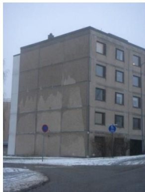
Fig. 5.15 End of a concrete building at the beginning of a rain event. The upper sections receive more rain than the lower ones.
