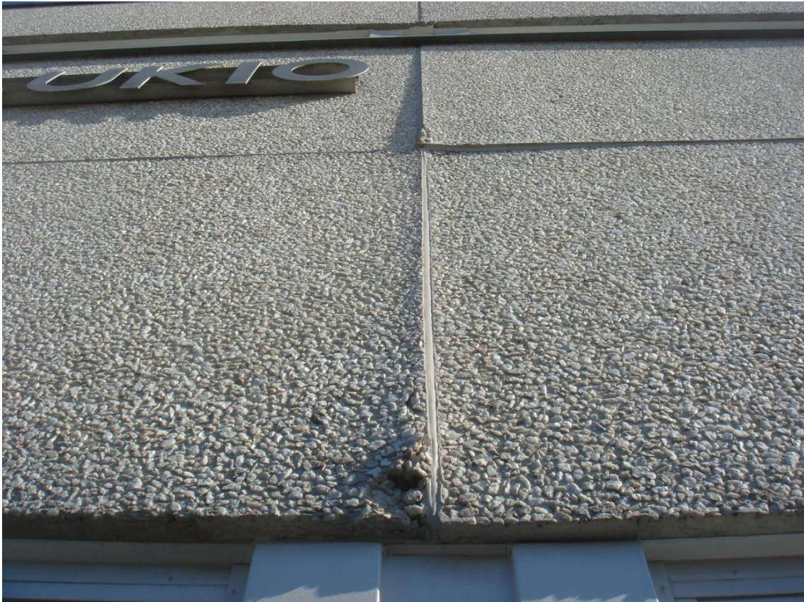
Fig. 2.2 Far advanced frost attack curls the edge of a facade panel.
