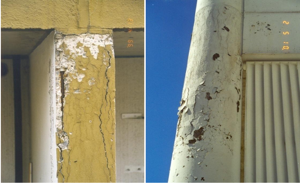
Fig. 5.26 On the left, local frost damage in the front edge of a balcony side panel. On the right, far advanced and extensive frost damage in balcony column. Both are load-bearing structures.
