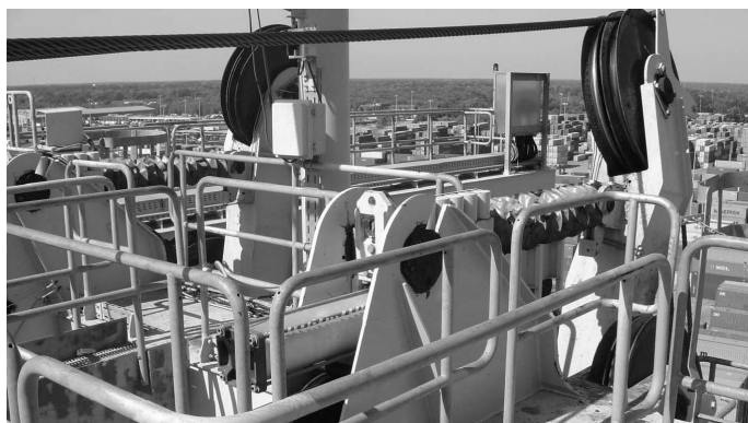
Figure 9.2 An example of a snag load system preventing excessive load peaks to lifting machinery and supporting structure. The operating principle of the system is based either on collapsible friction or hydraulic cylinders (Konecranes Plc).
