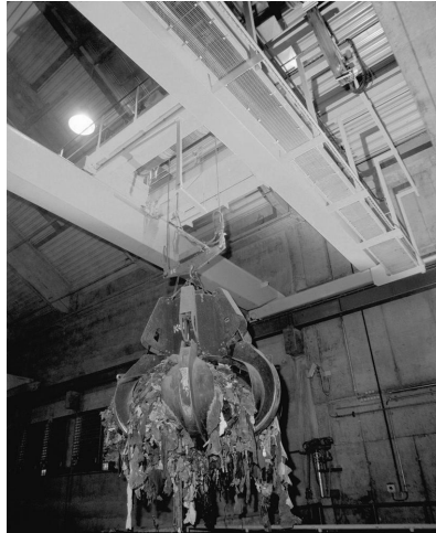
Figure 7.1 An overhead crane and hydraulic grab in waste-to-energy plant to move community waste from pit to oven (Konecranes Plc).
