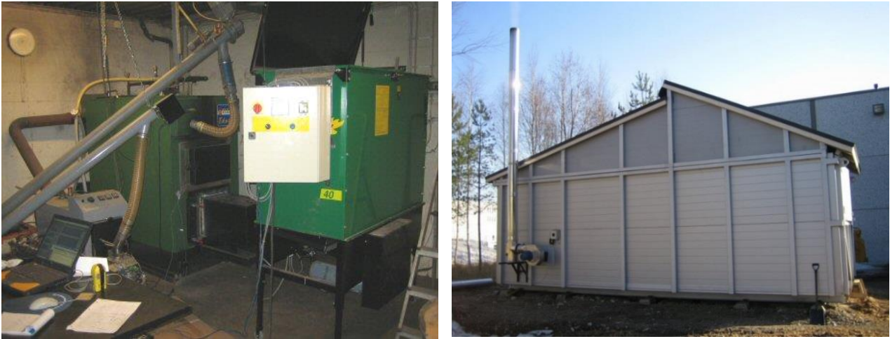
Figure 9. Left: 80 kW wood chip burner and 120 kW biomass boiler. (Korpela, 2006). Right: 200 kW heat container. The left side of the container constitutes of boiler room and the right side constitutes fuel storage. (Korpela & Björkqvist, 2008b)
