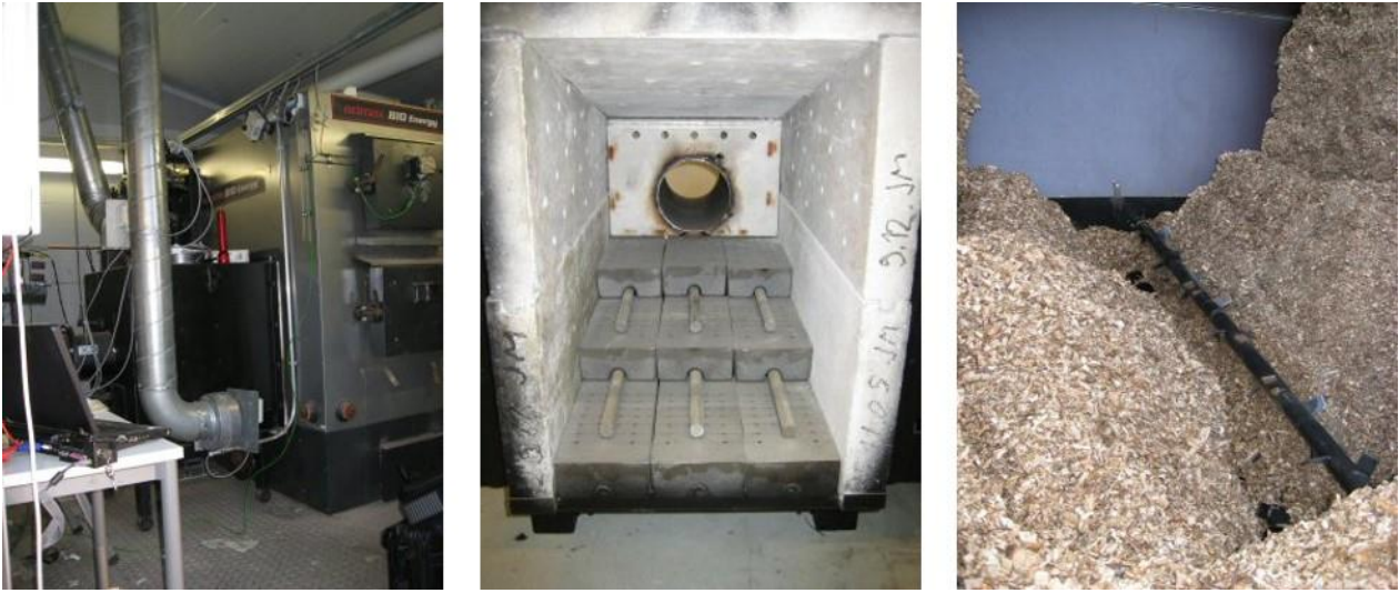
Figure 11. The 200 kW wood chip fired boiler. Left: Boiler room. Middle: Burner without the fuel feeding screw: Primary air feeds upward from the grate. Secondary air feeds from the walls and ceiling. The grate sweepers are at their outermost position. Right: Fuel feeding screw (lower) and auxiliary screw (upper) at partially revealed state in the fuel storage. (Korpela & Björkqvist, 2008b).
