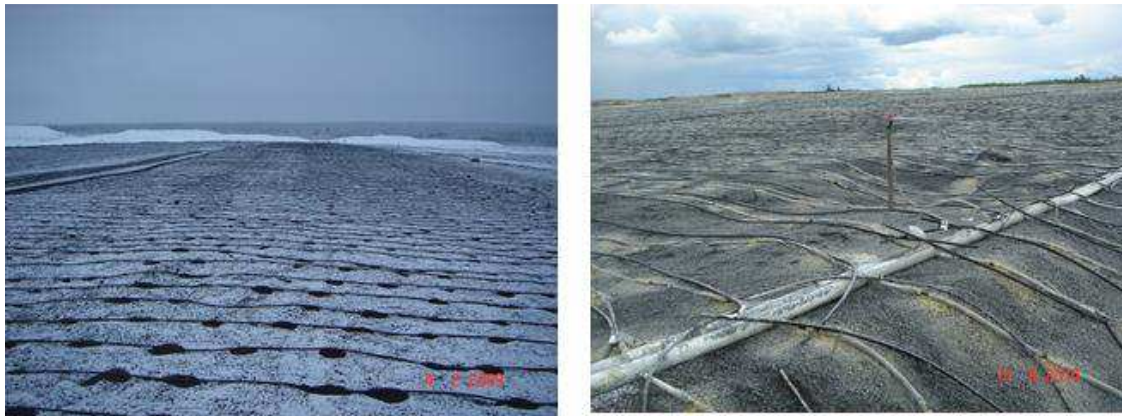
Figure 6. Photographs of the irrigation lines from Talvivaara bioheap. Photos: Marja Riekkola-Vanhanen.
