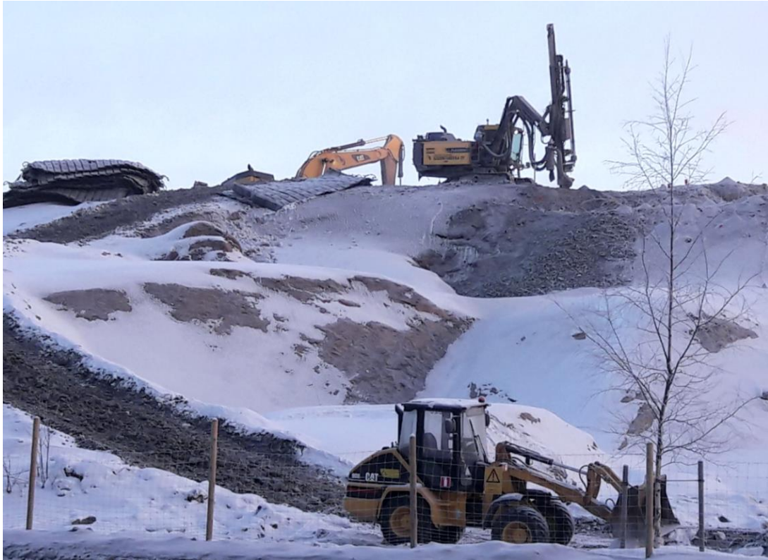
Figure 4.3. Tram line construction worksite in Tampere, in operation at -20 °C in Winter 2018.
