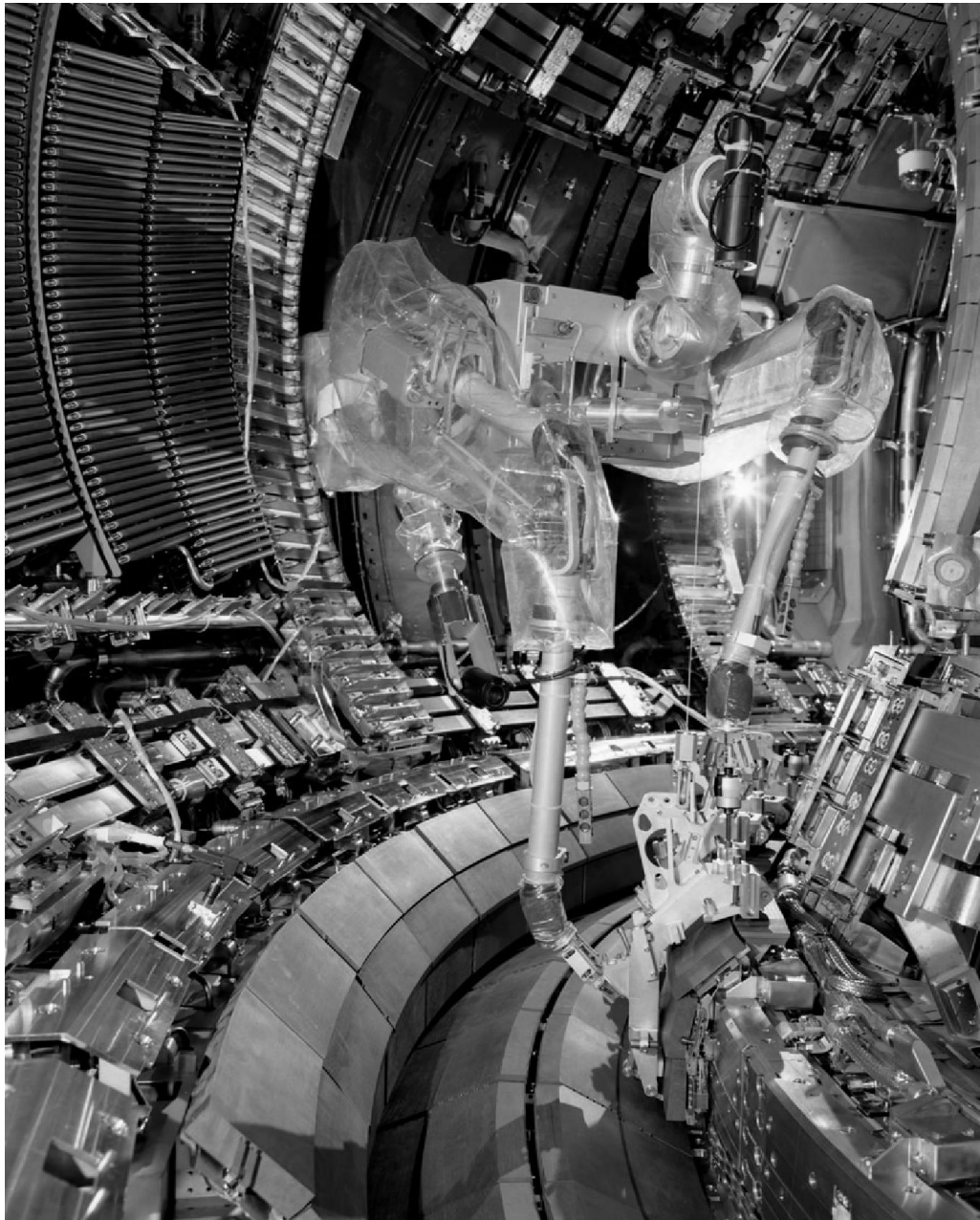
Figure 11: The Mascot manipulator inside the Joint European Torus removing a Divertor assembly using chest mounted winch, special Remote Handling compatible bolting tool and specially designed lifting jigs
