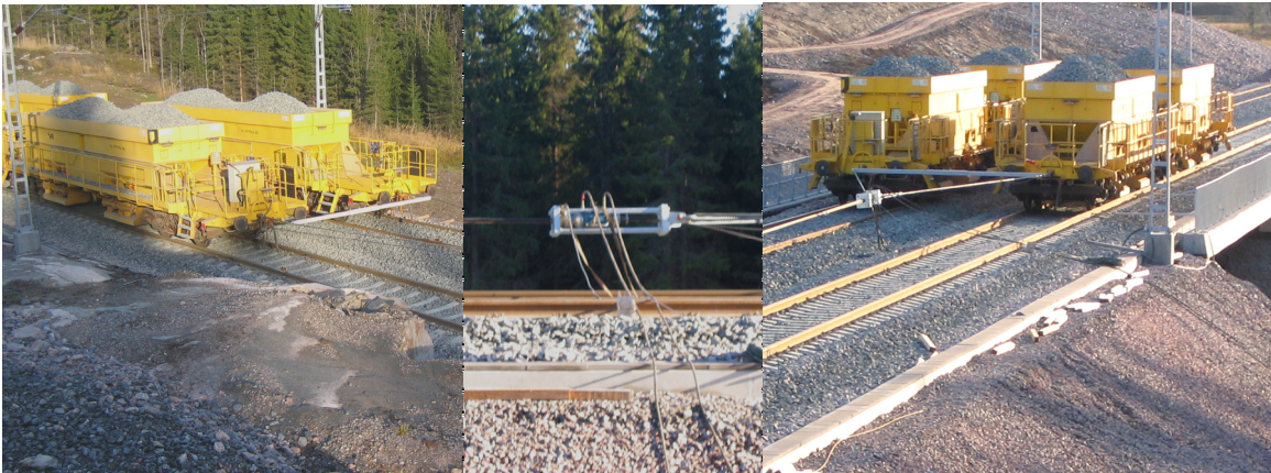
Figure 4.11. Load test at 30.10.2004 on the Tekemäjärvenoja Bridge site. On the left, counterweights. In the middle, post-tensioning jack with a load cell. On the right, railway waggons on the bridge.
