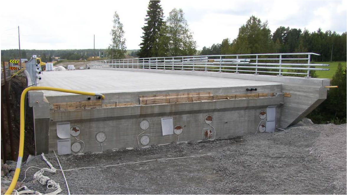
Figure 4.6. Installation of abutment EPCs, temperature gauges and gap measuring devices between the abutment and the embankment prior to approach fill construction. Anchor bars of end screen displacement measuring devices are also visible.
