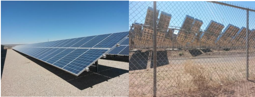
Figure 1.2. Solar panel installations in operation. On the left, Si flat panel installation connected to large batteries. On the right, an image of a 1 MW installation showing the back of the CPV panels. The panels are located in Albuquerque, New Mexico, USA.
